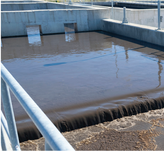
Sewage Treatment plant (STP)
